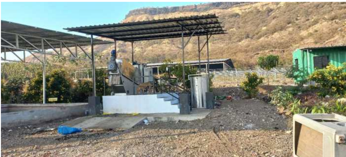
Pic. 7: Sludge treatment facility and drying bed
